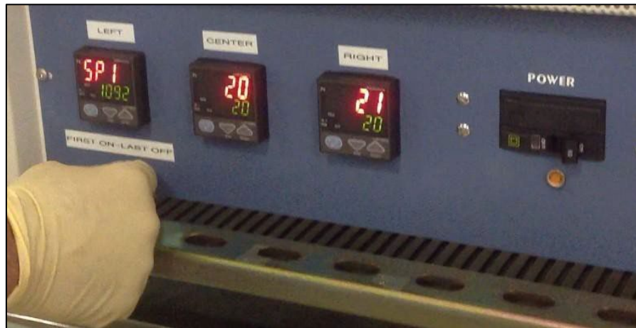
Figure 1 – Lindberg Temperature Controller Setup
